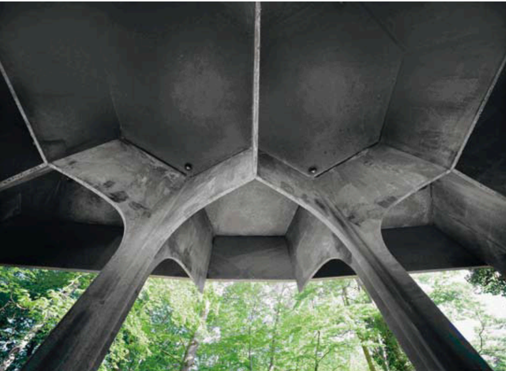
◀ FIG. 2 The first built example in the world using high-performance concrete internally cured by SAP addition: a pavilion in Kaiserslautern, Germany, constructed for the 2006 FIFA World Cup. //
